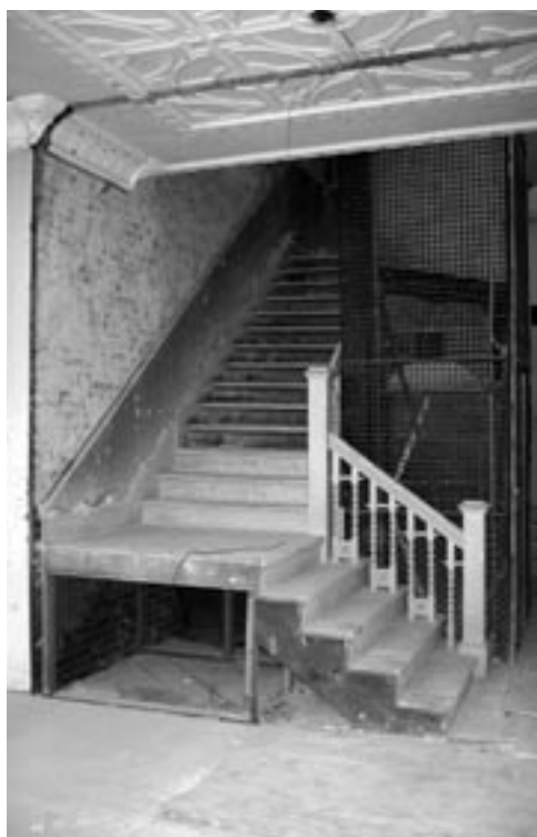
Light was shed on the original stairwell for the first time in over 25 years when the wall blocking it was re-opened.
