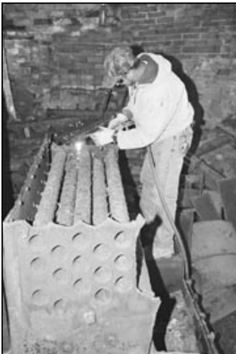
A blowtorch and two days time was needed to disassemble the original boiler in the Smith Center basement.
